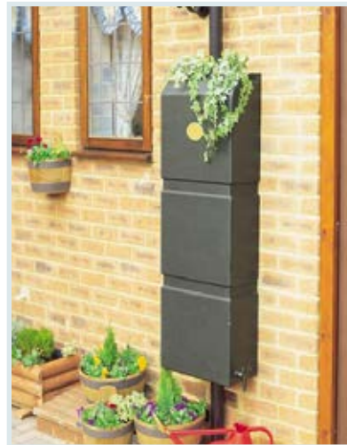
Figure 49: Example of a gravity-fed rainwater system for flushing a downstairs toilet or for irrigation.
